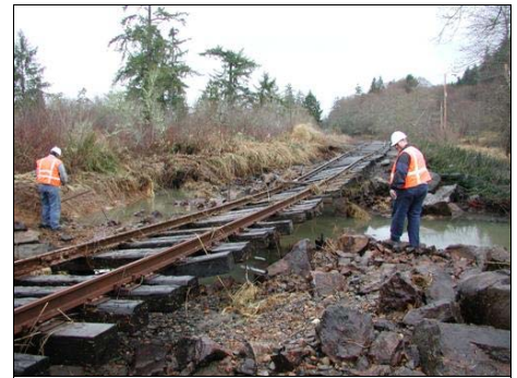
The railroad grade at Warren Slough was washed out in November 2006.
